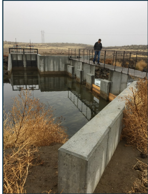
Figure 1: Diversion on Big Wood Canal similar in design to the proposed project. The proposed project will include the Constant Head Orifice Weir outlet structure only; the river-wide diversion will be excluded.
